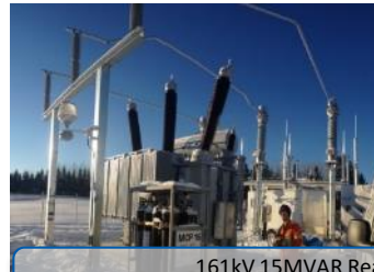
161kV 15MVAR Reactor Canada
